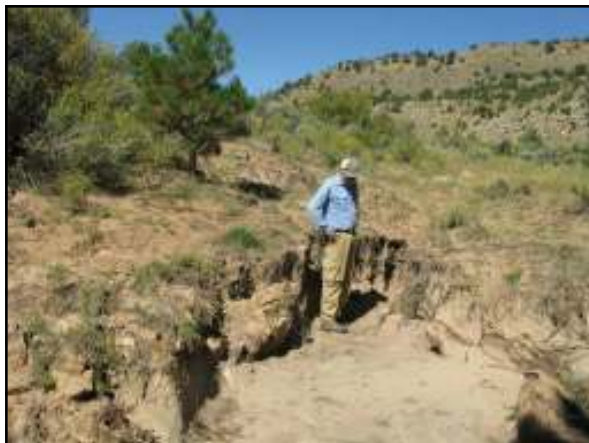
Lee Borduin checks out the remains of a portion of the Gallina River access road. These kinds of cuts are not unusual in the soft Gallina area soil.
