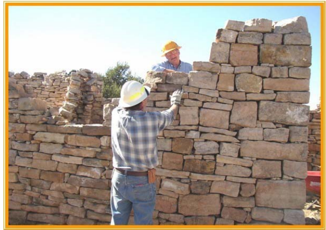
P.I.T. Volunteers working at the Hacienda Site All Photos by Brent Abel
