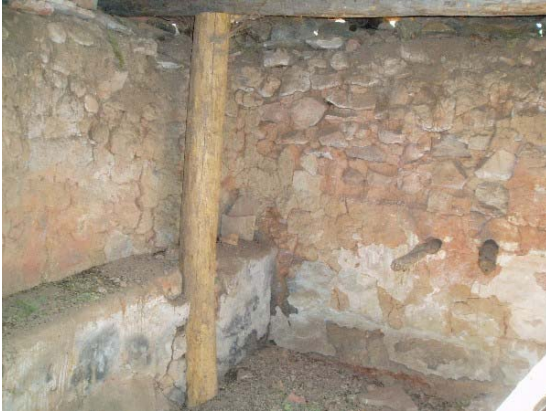
Preserved and covered unit house demonstrates charred plaster on walls indicating site had been burned with extreme heat.
